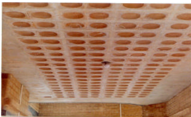
Figure 8. Ceiling of a typical filler slab roof using stabilized mud block filler.
